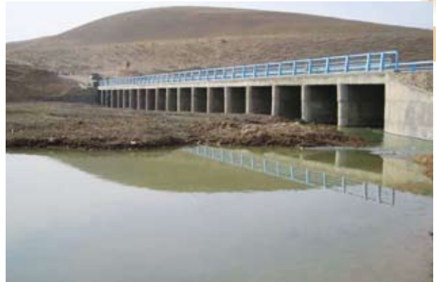
Bridge built by Badghis PRT, allowing military and civilian economic development teams to reach remote areas.
