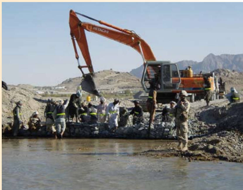
Construction of a causeway across the Arghandab River between the districts of Zhari and Panjwayi.
