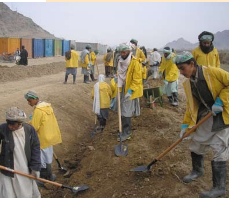
Local workers undertake the construction of the 6.5 Km road to Panjwayi district centre.
